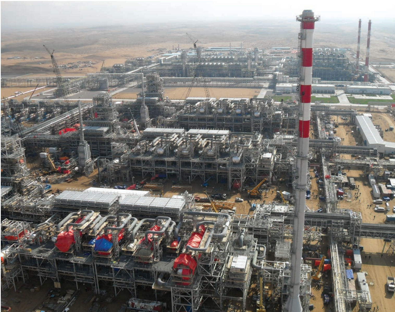
Galkynysh Gas Field Development, Turkmenistan
